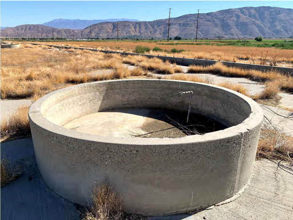
G-2. Abandoned concrete improvements in the southeastern corner of the Site related to former heifer ranch operations (08/03/2021).
