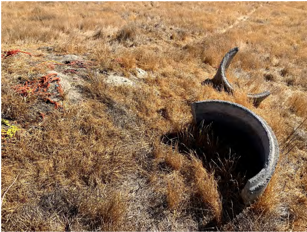
G-3. Miscellaneous concrete debris in southeastern corner of the Site (08/03/2021).
